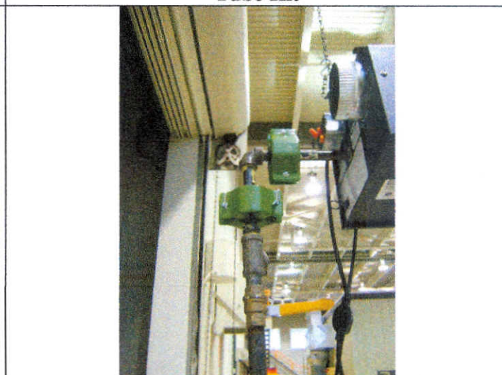
Get Green Device, installed
